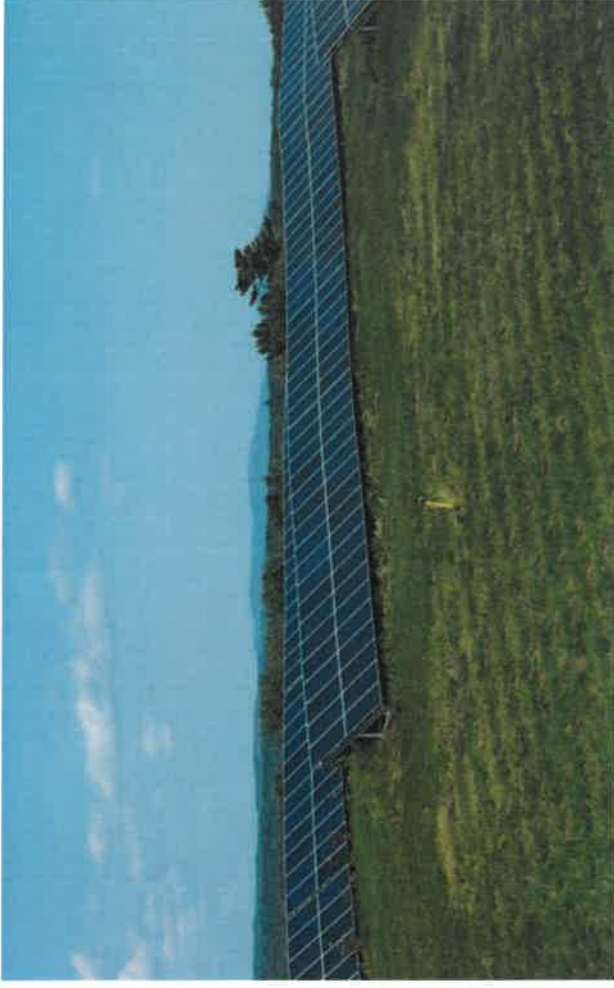
Solar array on the top of Waldoboro's capped landfill
